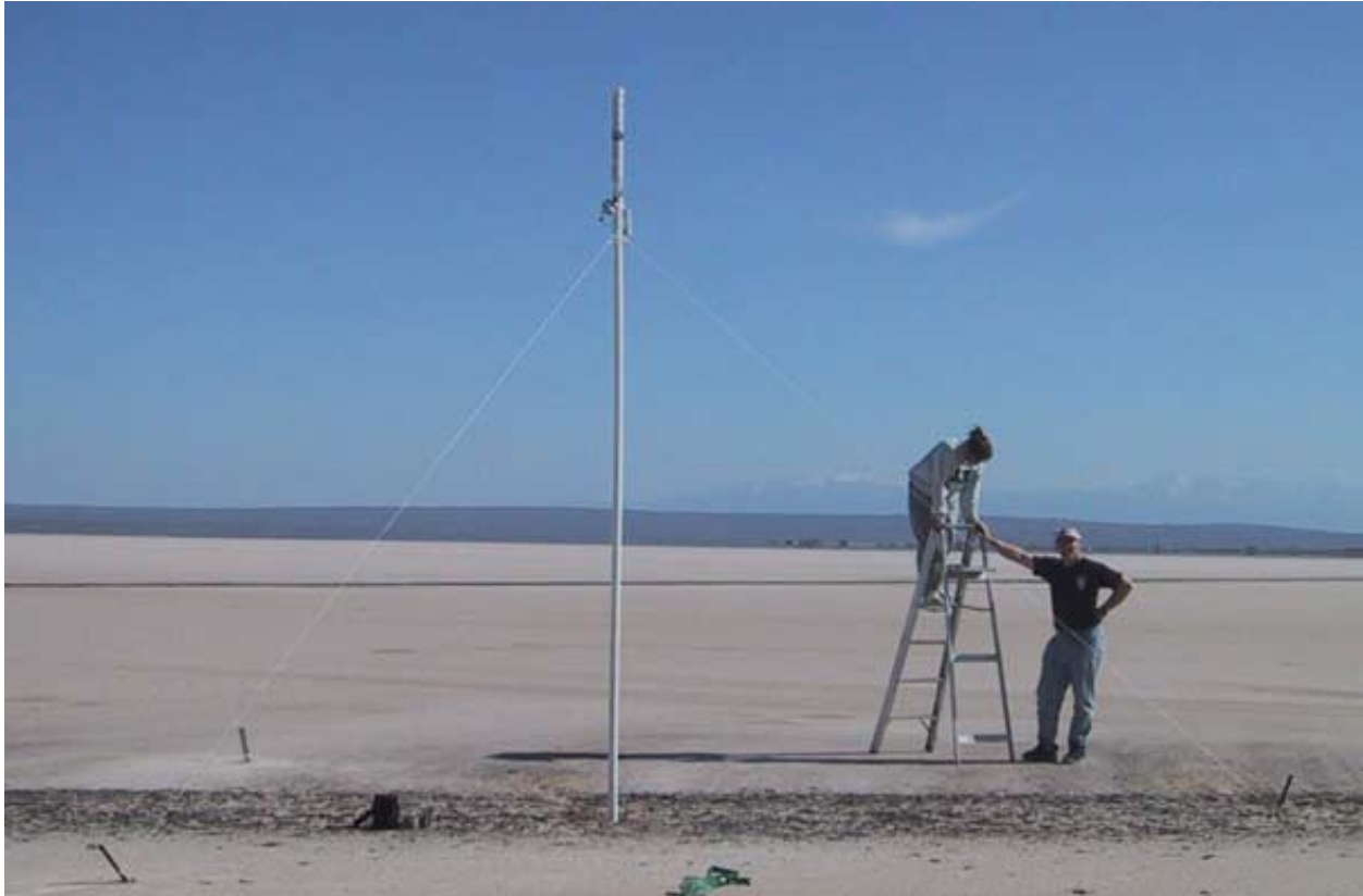
Figure 10. Installed Test Antenna In “Zero-Coax” Feedline Configuration
