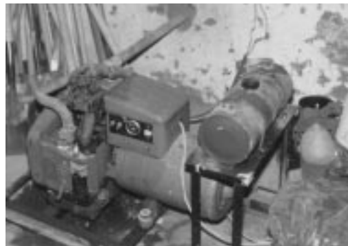
Figure 3.8. Typical generator at an isolated mountain school. Teachers and custodians generally have no training in the maintenance and operation of these units.
