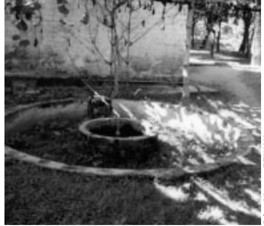
Figure 6.9. Biogas plant digester.
